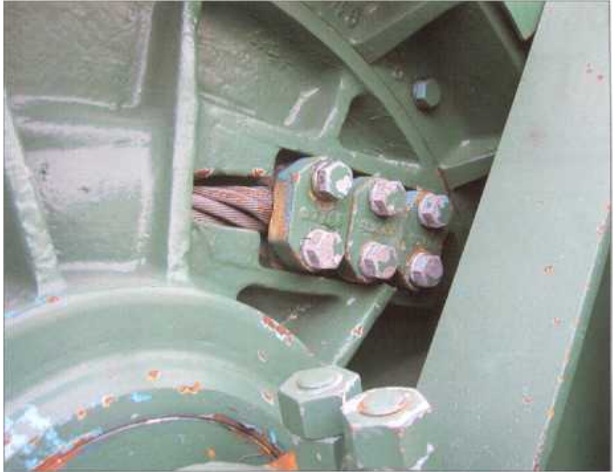
This is a custom, triple-plate termination. Photo by Barry Griffin.
